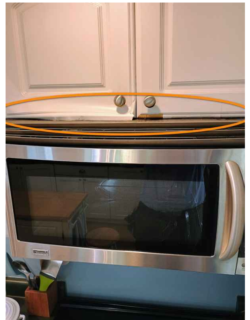
Thermofoil cabinet doors show delamination
