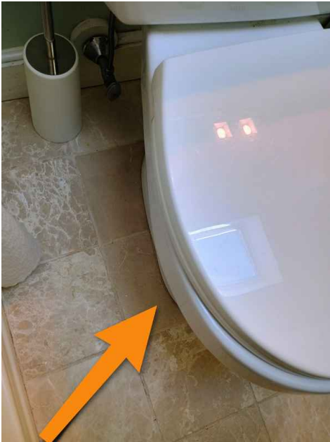
Toilet was loose on its moorings
