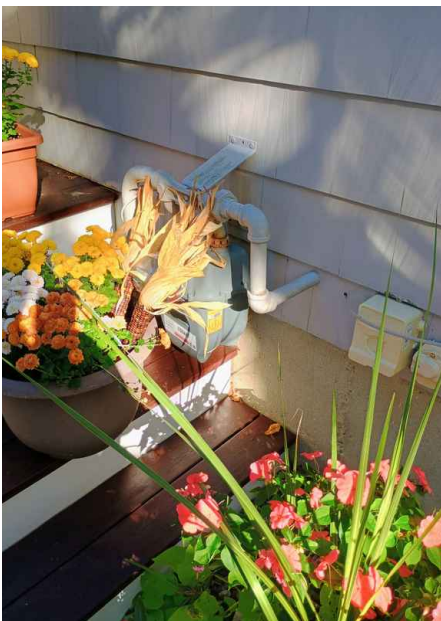
Gas meter at mudroom entrance
